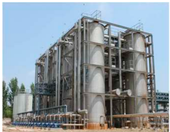
Fig 2: Industry: Textile Central Effluent Treatment Plant, Capacity: 180 MLD
